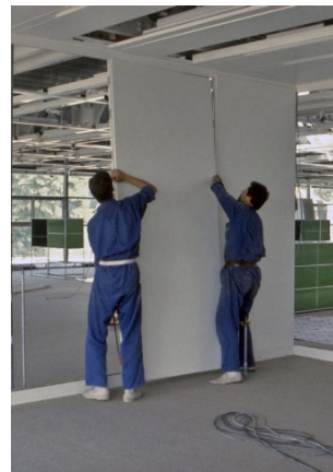
Figure 1 and 2: Component System MIDI, Training center of swiss federal railways (SBB) in Löwenburg Murten Switzerland, 1980-82, Fritz Haller
